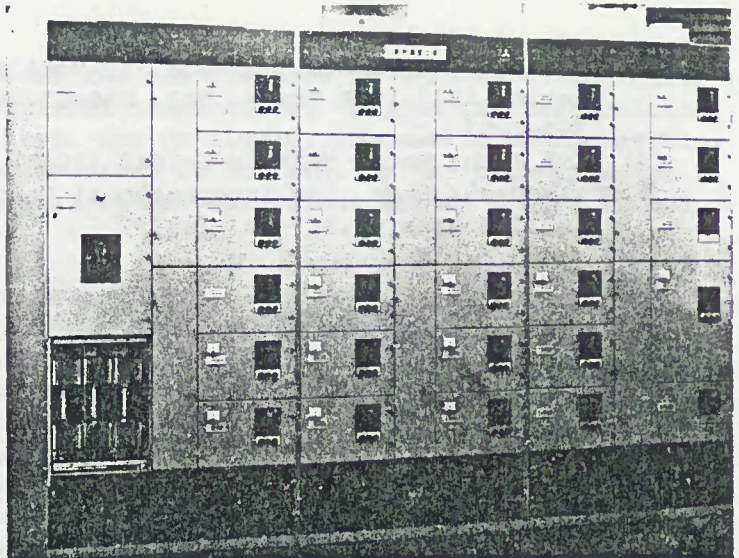
Fig-2. Outside view of the PPFused control center
